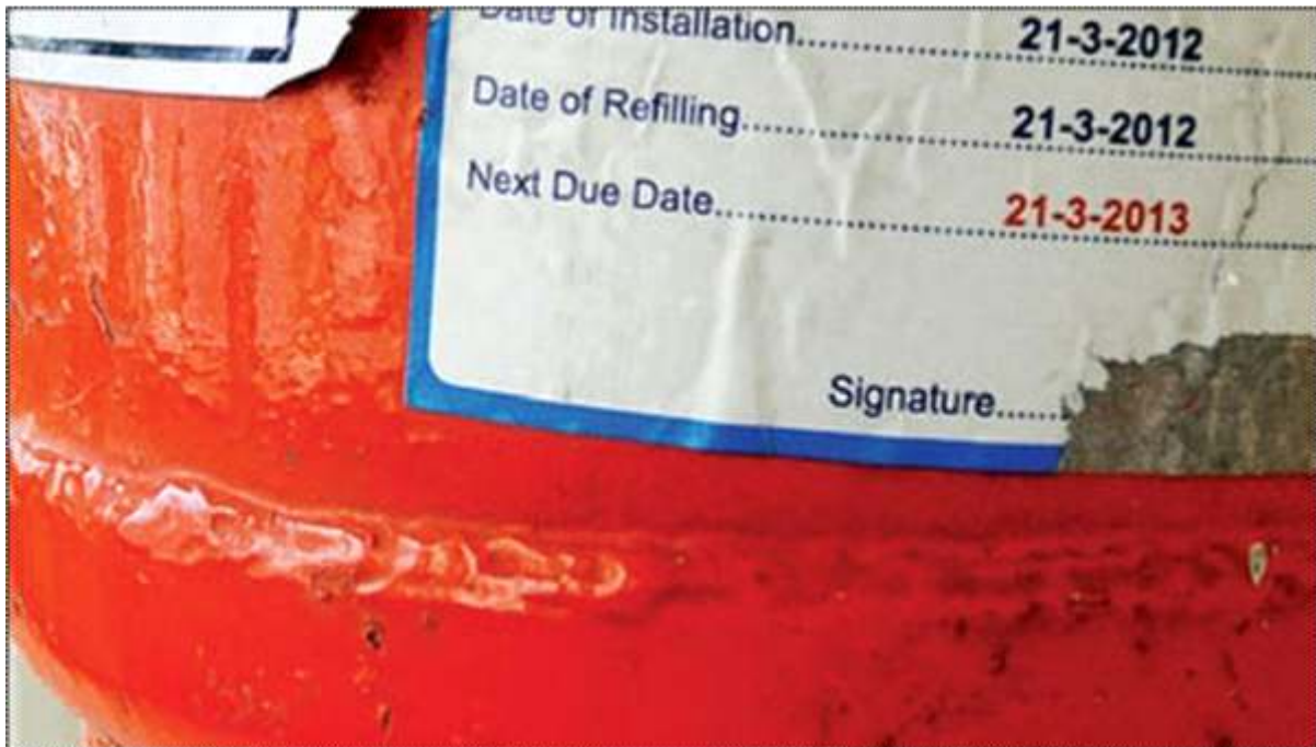
Fig 8.4.1.3 Know the refill date on the fire extinguisher
